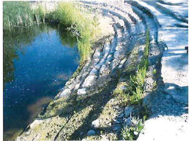
Photo 2 - Typical Seepage Thru Structure
