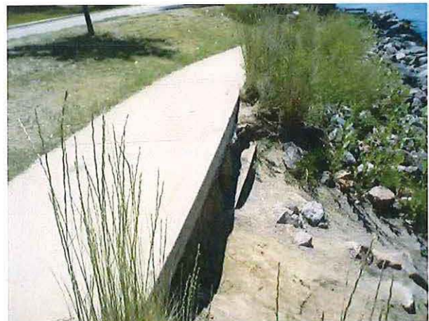
Photo 27 – Shoreline Erosion along Walkway
