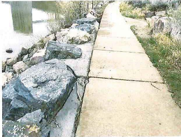
Photo 31 - Tower Loop Shoreline Erosion at Access Walk
