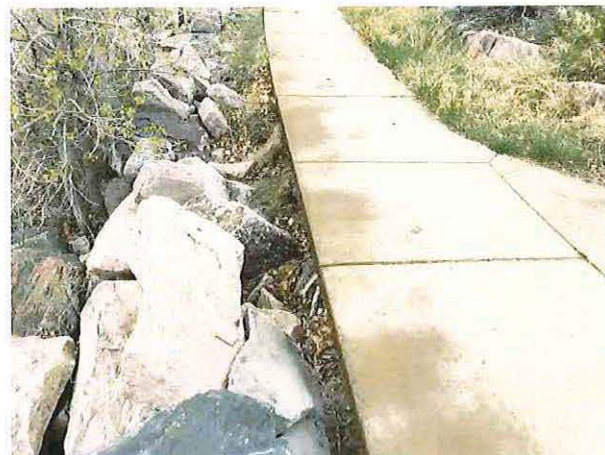
Photo 30 - Tower Loop Shoreline Erosion at Access Walk
