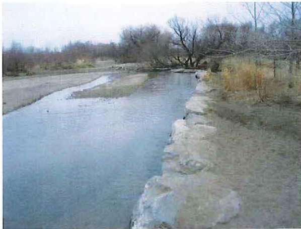
Photo 12 - 12-Mile Park, Phase I Channel Sediment Aggradation
