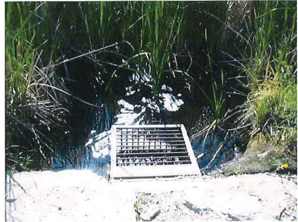
Photo 4 - Typical Inlet Trash Rack
