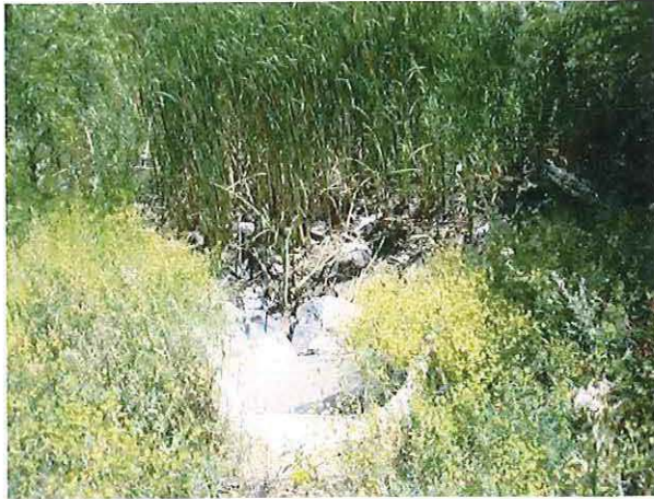
Photo 34 – WBR Pipe Inlet Flared End Section
