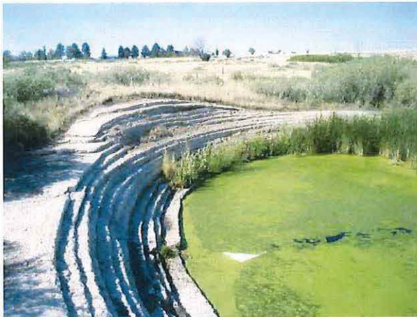
Photo 1 - Typical Structure Deterioration
